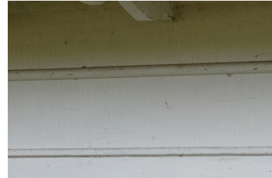
17. Peeling paint, west extension.
