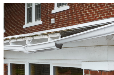
21. Damaged south gutter.
