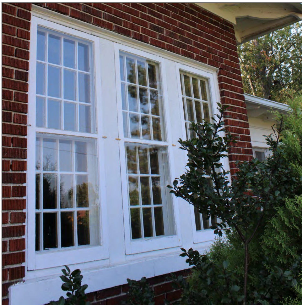
Figure 21: Detail view of a first-floor window on the front of 183 Main Street East (Source: ML, 2020).
