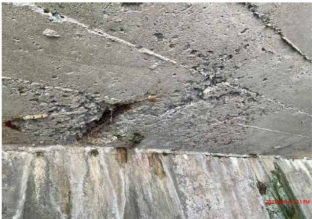
Photo 18 Concrete delamination and exposed corroded steel reinforcement in deck soffit adjacent to west abutment.
